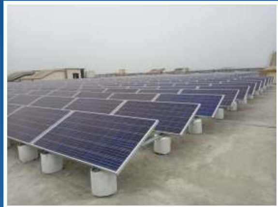
Capacity : 1Mw (Consolidated) Year : 2018
