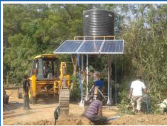
Project : PHED, Bankura Type : Solar Powered Pump with hand pump system
