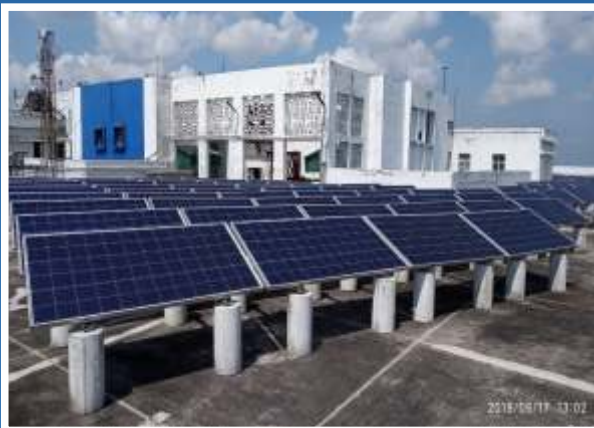
Project : WBSEDCL Type : Grid Connected (Roof top)
