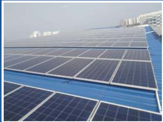
Capacity : 100 KWp Year : 2019
