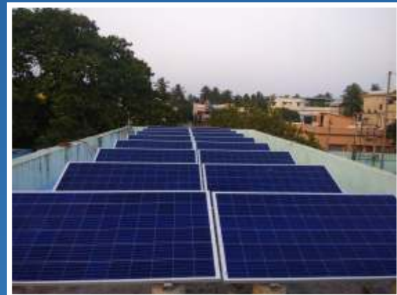
Capacity : 350 KWp (Consolidated) Year : 2019
