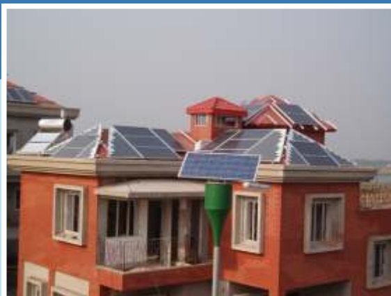
Project : Rabi Rashmi Abashan Type : Grid Connected BIPV System
