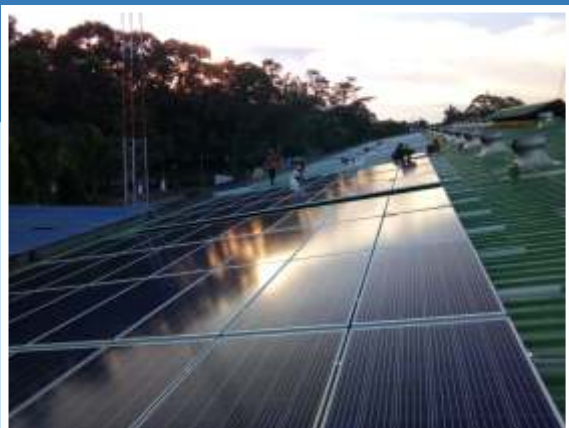
Project : TGBL, Assam Type : Grid Connected (Roof top)
