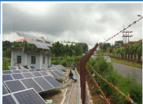
Project : SPV Power Plant at NEHU, Shilong Type : Off Grid
