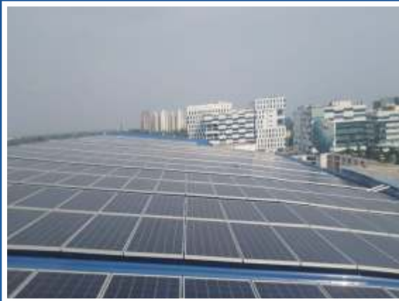
Project : IIIT, Newtown, Kolkata Type : Grid Connected (Roof top)
