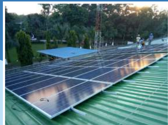
Capacity : 210 KWp (Consolidated) Year : 2019
